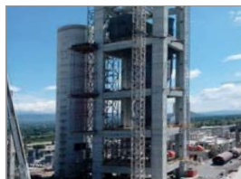
Clinker Production Line
